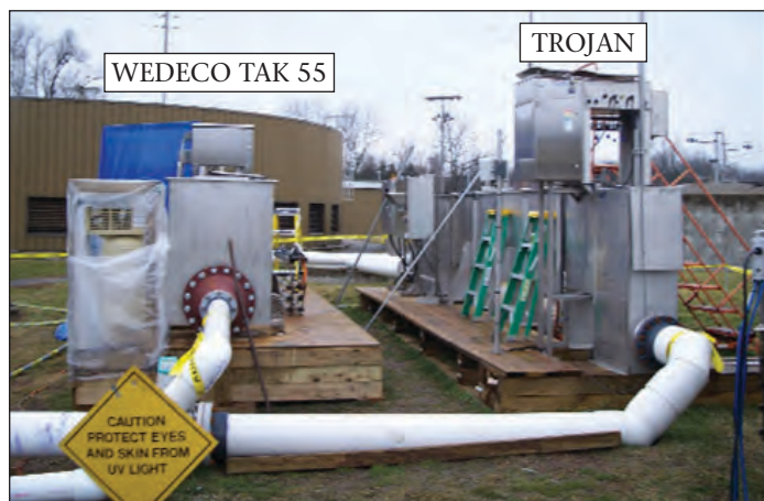
Figure 3. UV Pilot Systems
