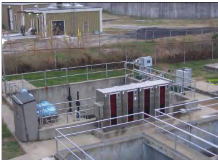
Figure 1. Olathe UV System
