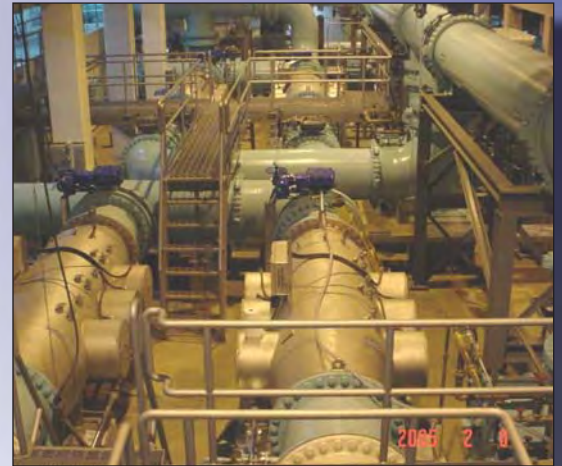
UV Disinfection Facility at the Water Treatment Plant in Winnipeg, MB, Canada (130 MGD)
