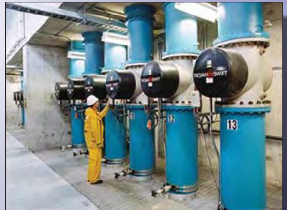
UV Disinfection Facility at the Water Treatment Plant in Seattle, WA (180 MGD)
