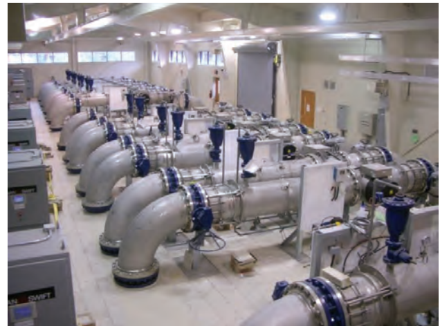
Figure 4. UV reactors and headers installed
