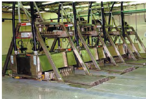
Trojan System UV4000™; 4 channels, 150 MGD flow rate
