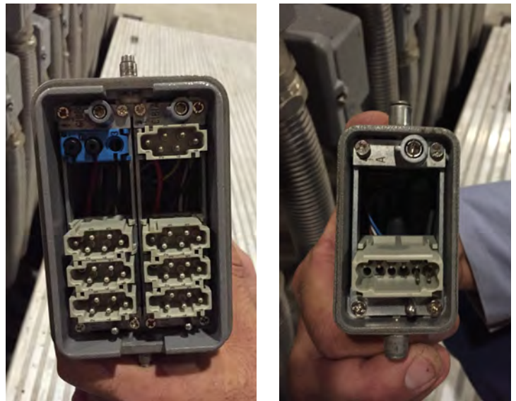
Figure 3. Loose lamp and sensor cable connections
