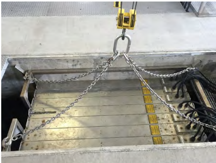
Figure 4. Clearance issues when removing modules
