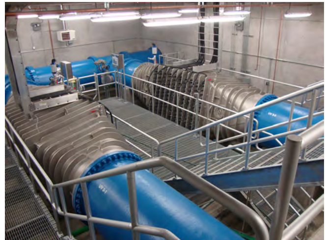
Figure 4. Photograph of the low-pressure, high-output UV reactors at a SWD UV disinfection facility.
