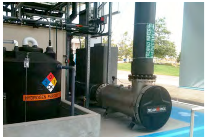
Figure 3. San Diego, CA UV System that is Part of the Water Purification Demonstration Pilot
