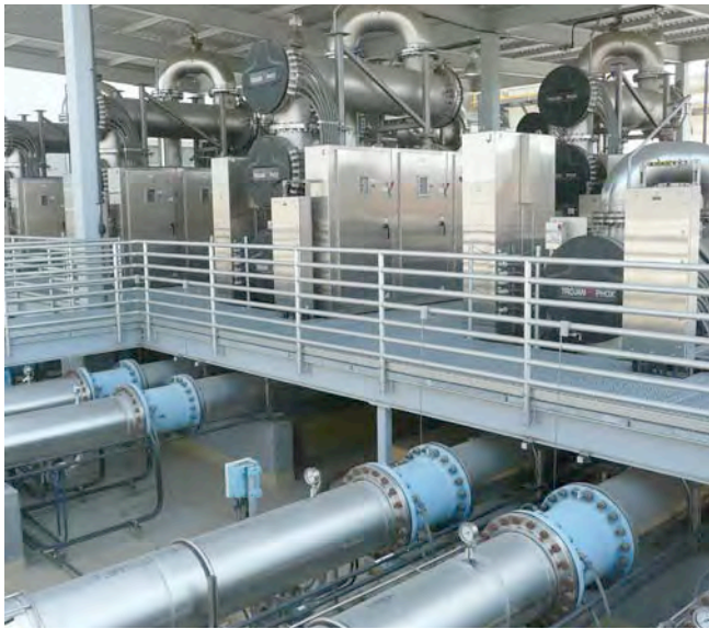
Figure 2. Orange County, CA Groundwater Replenishment System UV Process
