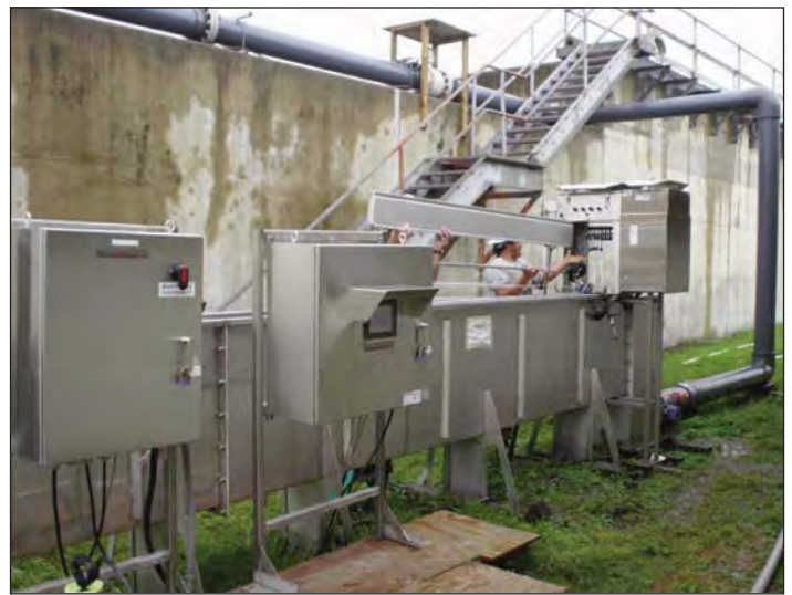
Figure 4: Photograph of On-site Fouling Factor Pilot Unit
