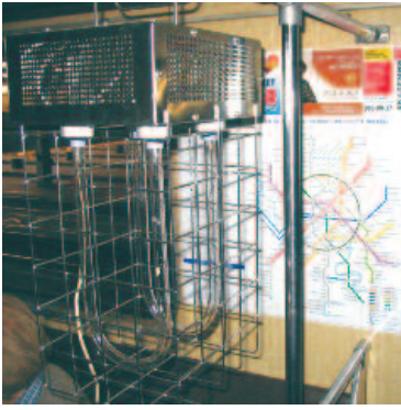
Figure 6. UV system for interior disinfection, with two U-shaped 170 W UV lamps.
