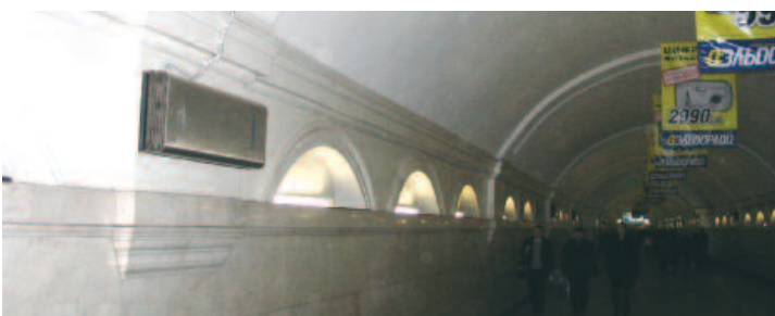
Figure 9. Recirculator AR-UF-170-2 mounted in the passage between “Paveletskaya-Radial’naya” and Paveletskaya-Koltsevaya”.
